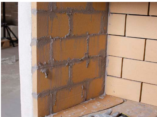
Use the mortar mix to point up the joints between the firebricks once they are all in position.
